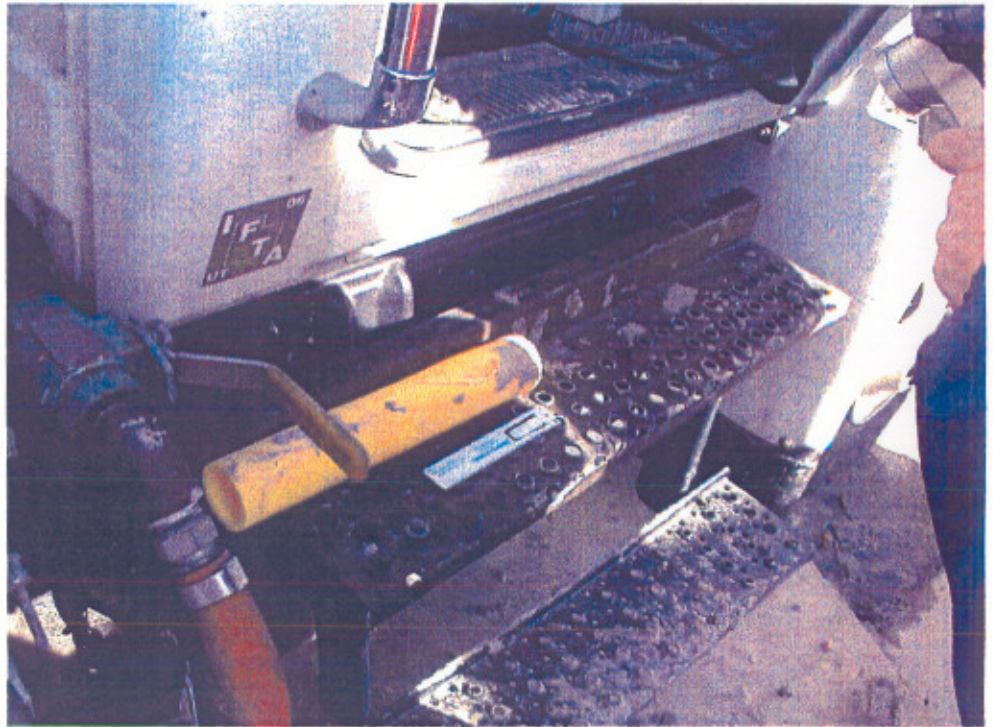
#30 Damaged section of the main, 02/07/07
