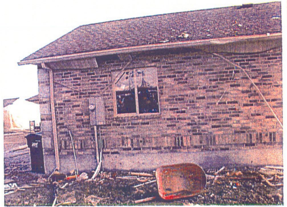
#18 Damage to W. of adjacent home at 953 W. Prairie Dog Way, 02/07/07
