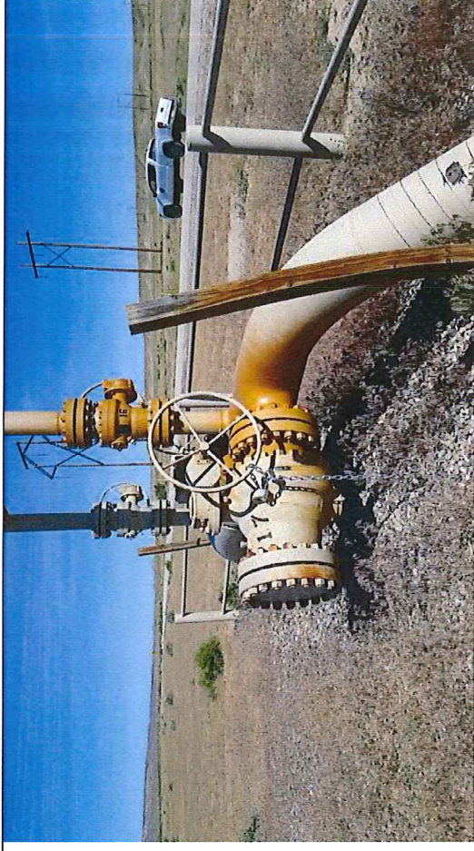
Picture #6: Block Valve assembly BV-14, BV-15, BV-16, and BV-17.
