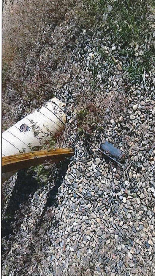
Picture #8: Observed Corrosion Protection SSD (Solid State Decoupler) dismounted from the pole.
