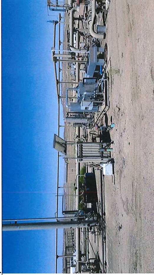
Picture #23: Observed PEMC compressor station with BV-2 in the open position.
