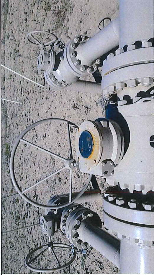
Picture #21: Observed valve assembly east of PEMC compressor station with BV-3 and BV-4 in the close position and BV-2 in the open position. All valves chained and locked.
