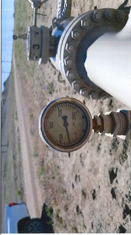
Picture #22: Pressure gauge near BV-3 on the gathering side, approximately 250 psig.
