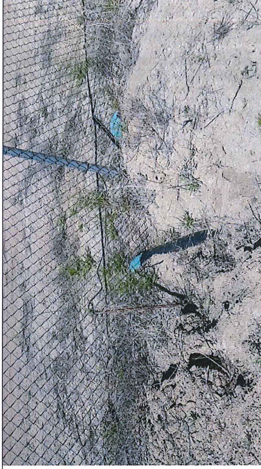
Picture #24: Observed PEMC compressor station exposed piping near the east fence.
