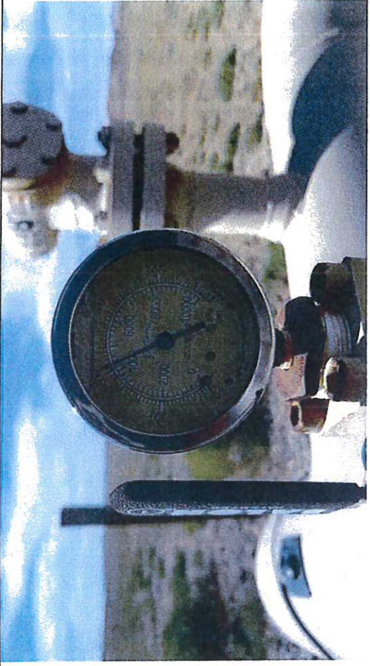
Picture #26: Pressure gauge near BV-7 approximately 610 psig.
