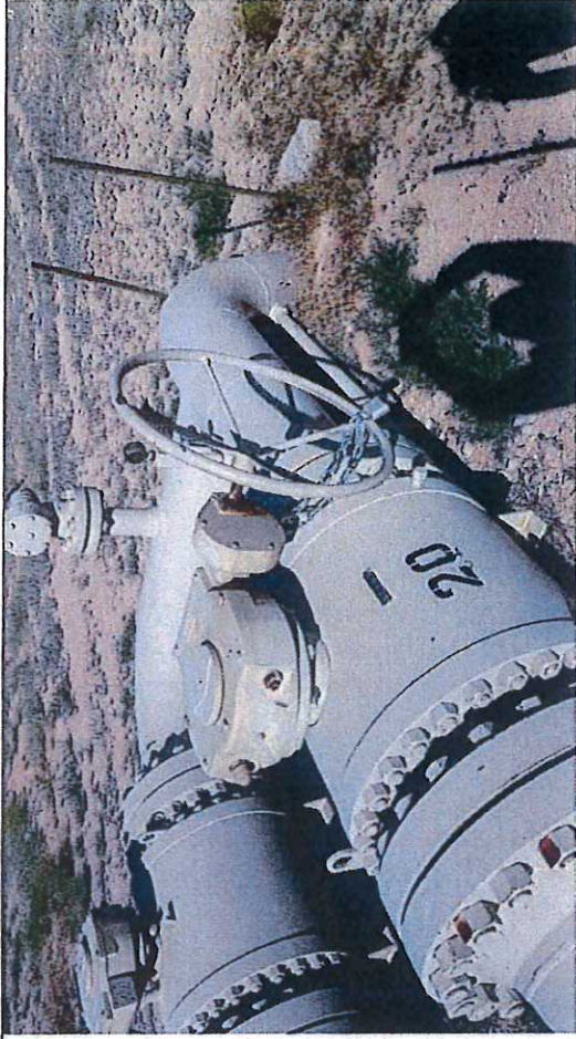
Picture #4: Block Valve BV-20 and BV-19 (vent), observed close position with chain and lock.
