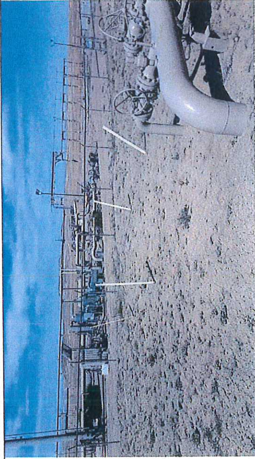
Picture #27: Observed valve assembly east of PEMC compressor station.
