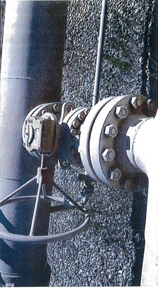
Picture #18: Block Valve BV-6, observed in close position with chain and lock.
