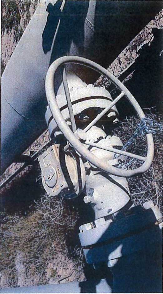
Picture #2: Block Valve BV-21, observed in close position with chain and lock.
