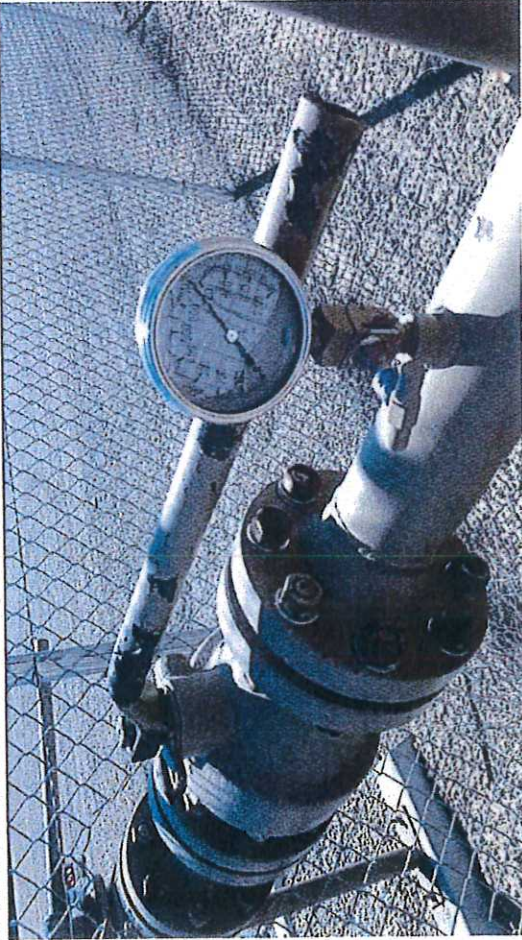
Picture #13: Observe Wesco Compressor Station at Blue Hills PEMC Valve open position.
