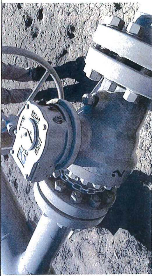
Picture #32: Block Valve BV-2, observed in close position with chain and lock.
