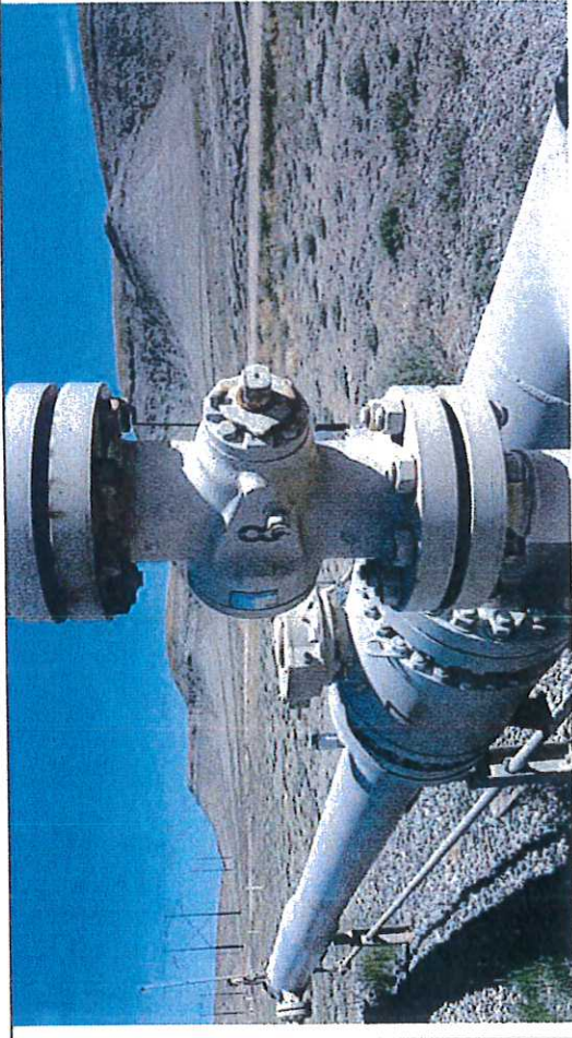
Picture #25: Block Valve BV-8, observed in close position with chain and lock.
