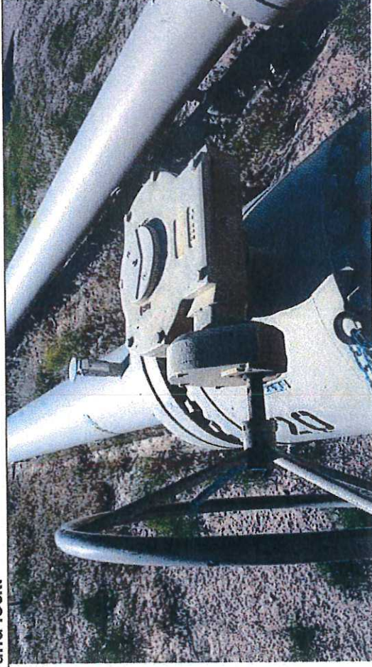
Picture #3: Block Valve BV-20, observed in close position with chain and lock.
