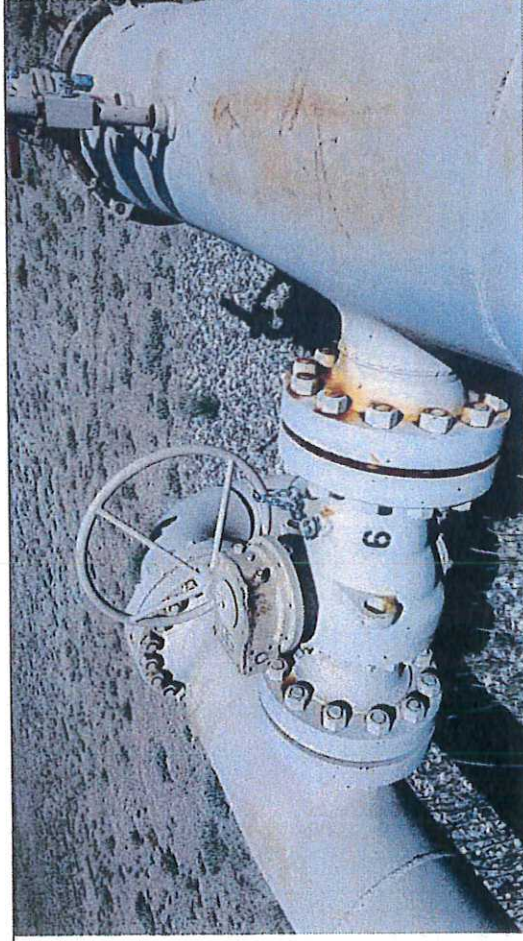
Picture #23: Block Valve BV-6, observed in close position with chain and lock.
