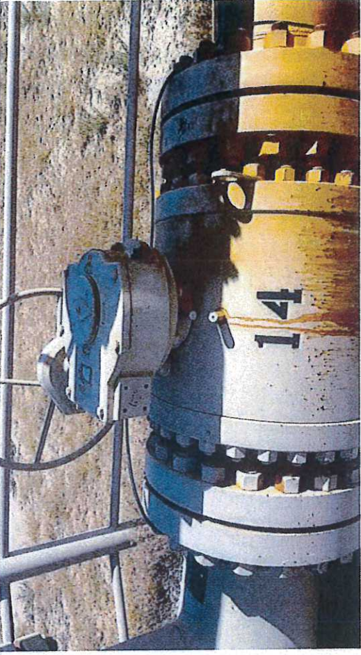
Picture #6: Block Valve BV-14, observed in close position with chain and lock.
