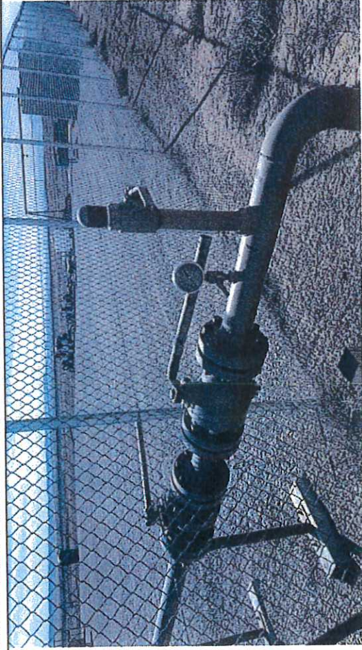
Picture #18: Observe Wesco Compressor Station at Blue Hills, PEMC Valve open position.
