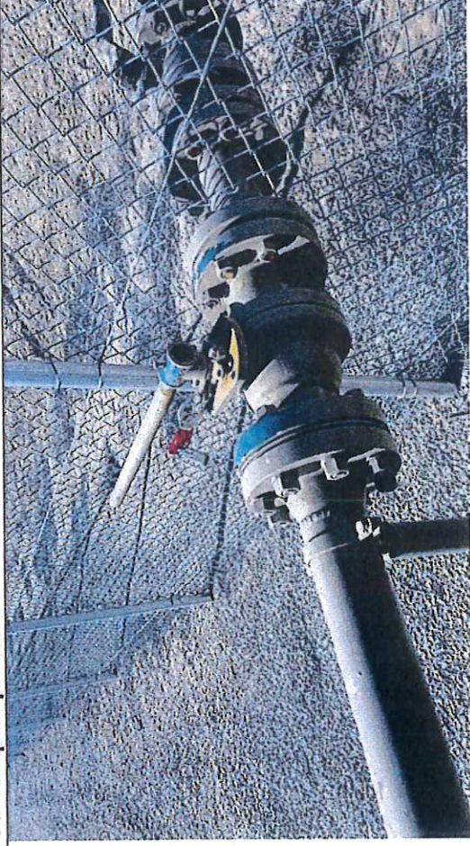
Picture #15: Observed Wesco Compressor Station at Blue Hills Wesco valve close position.
