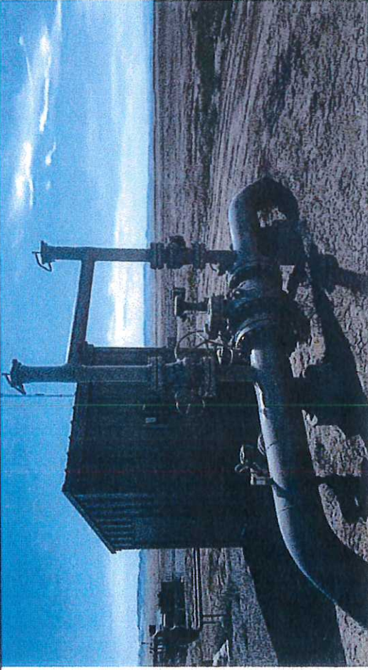
Picture #10: Wesco Tie-In Point at Blue Hills Station.
