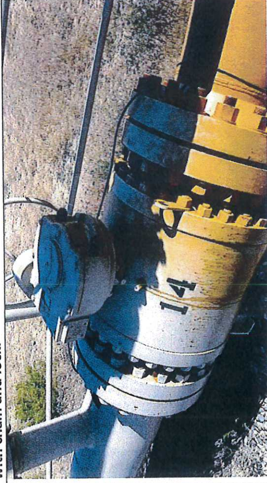
Picture #7: Block Valve BV-14 north side, observed in close position with chain and lock.
