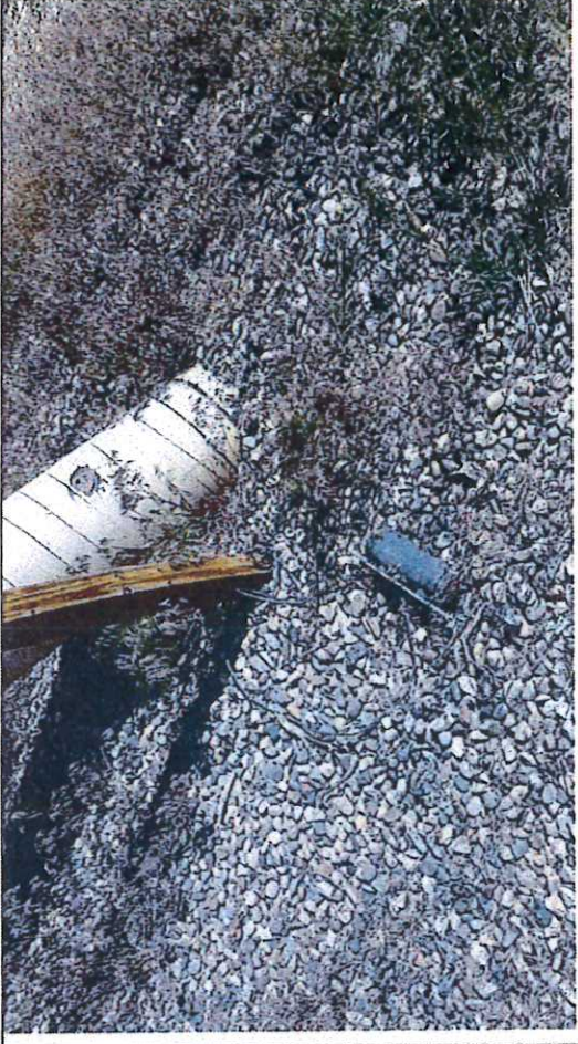
Picture #8: Observed Corrosion Protection SSD (Solid State Decoupler) dismantled from the pole.
