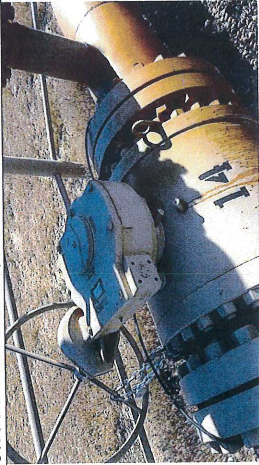
Picture #5: Block Valve BV-14 south side, observed in open position with chain and lock.
