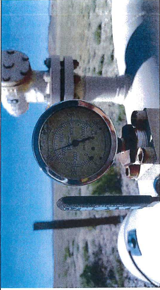
Picture #20: Pressure gauge near BV-7 approximately 680 psig.
