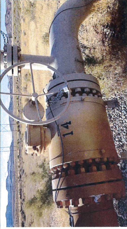
Picture #10: Block Valve BV-14, observed in close position with chain and lock.
