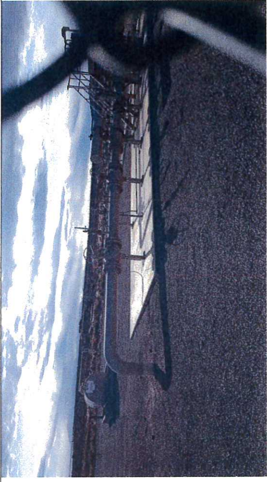
Picture #8: Aboveground piping in the Northwest William Pipeline Tie-In yard.
