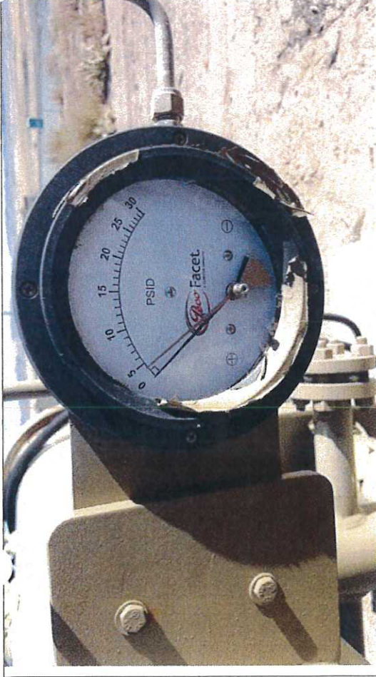
Picture #22: Wesco Gathering Side Pipeline Gauge Pressure, observed 0 psig.
