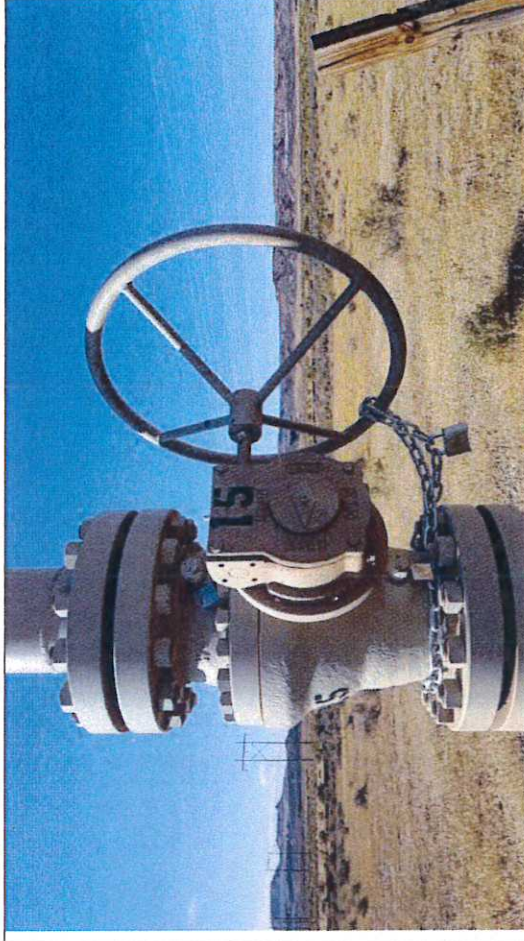
Picture #12: Block Valve BV-15, observed in close position with chain and lock.
