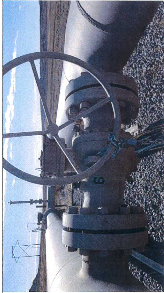
Picture #30: Block Valve BV-6, observed in close position with chain and lock.
