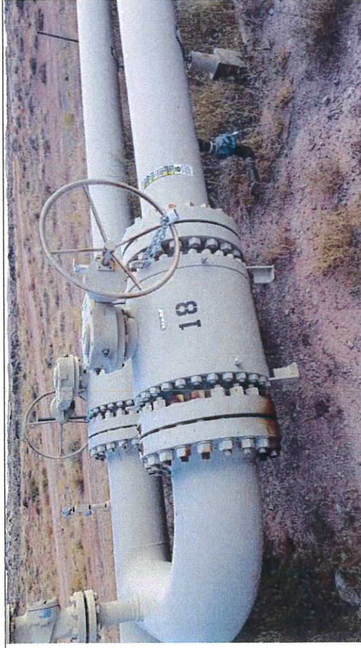
Picture #3: Block Valve BV-18, observed in close position with chain and lock.
