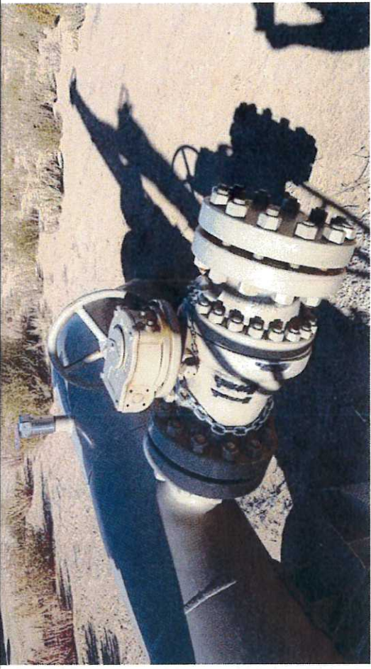
Picture #17: Block Valve BV-11, observed in close position with chain and lock.
