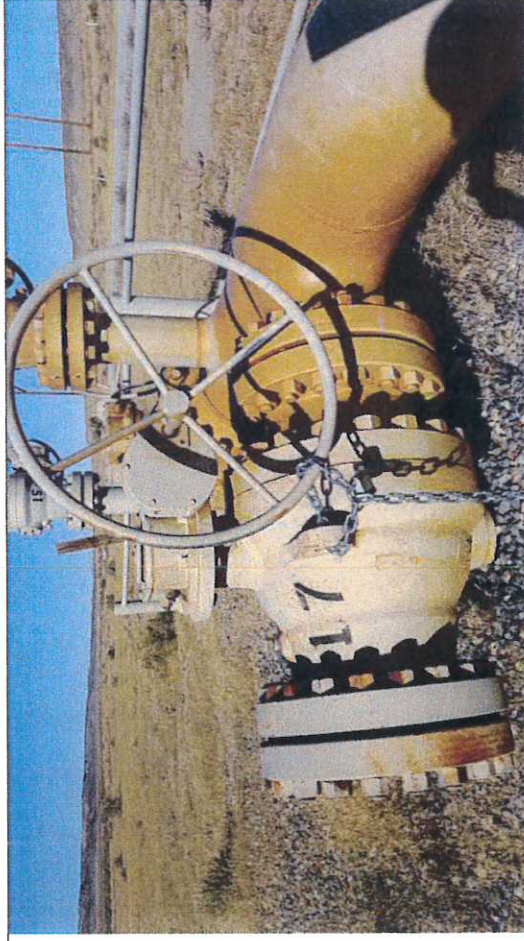
Picture #11: Block Valve BV-17, observed in close position with chain and lock.
