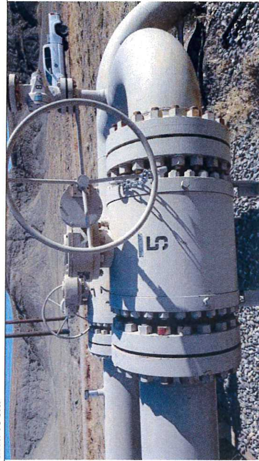
Picture #31: Block Valve BV-5, observed in close position with chain and lock.
