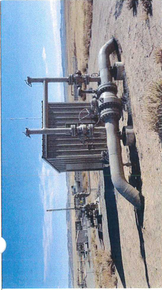
Picture #14: Wesco Tie-In Point at Blue Hills Station.
