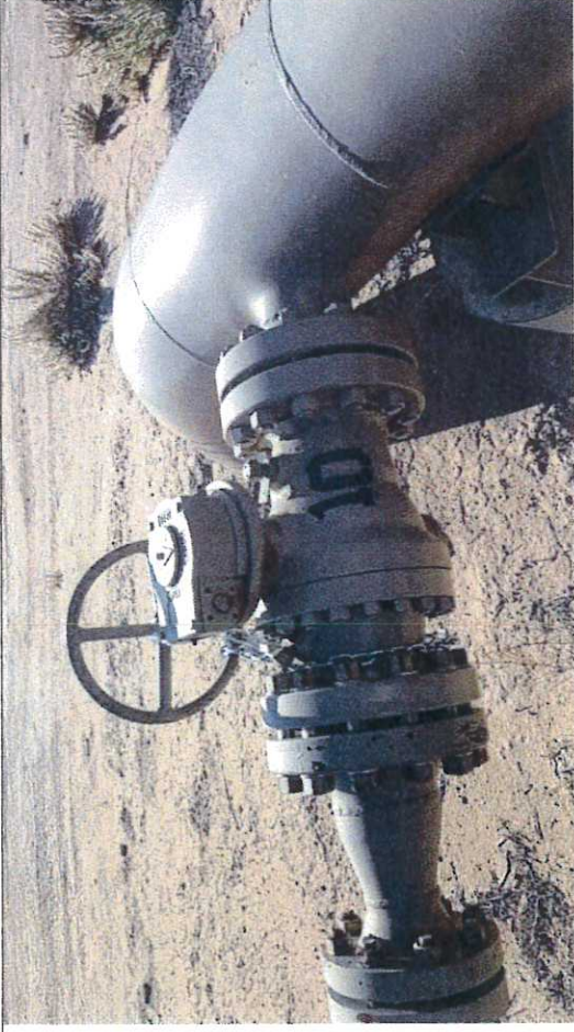
Picture #16: Block Valve BV-10, observed in close position with chain and lock.
