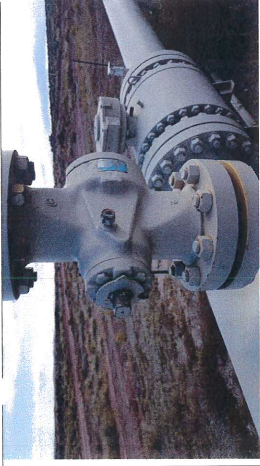
Picture #5: Block Valve BV-19 (Blowdown Vent), observed in close position.
