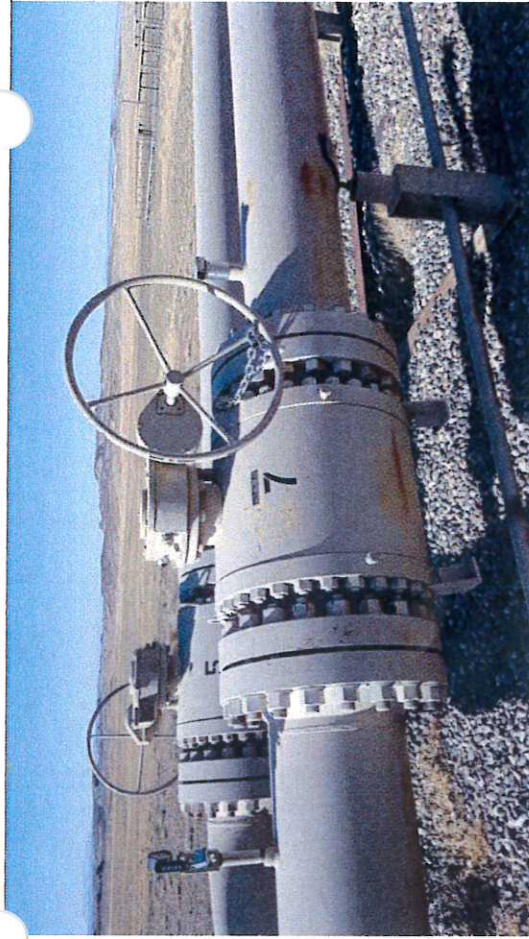
Picture #29: Block Valve BV-7, observed in close position with chain and lock.
