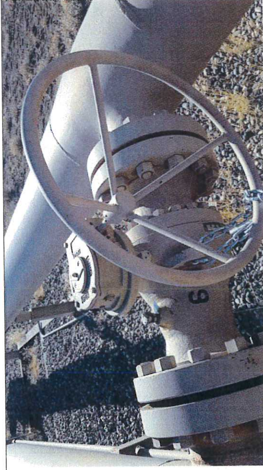
Picture #30: Block Valve BV-6, observed in close position with chain and lock.
