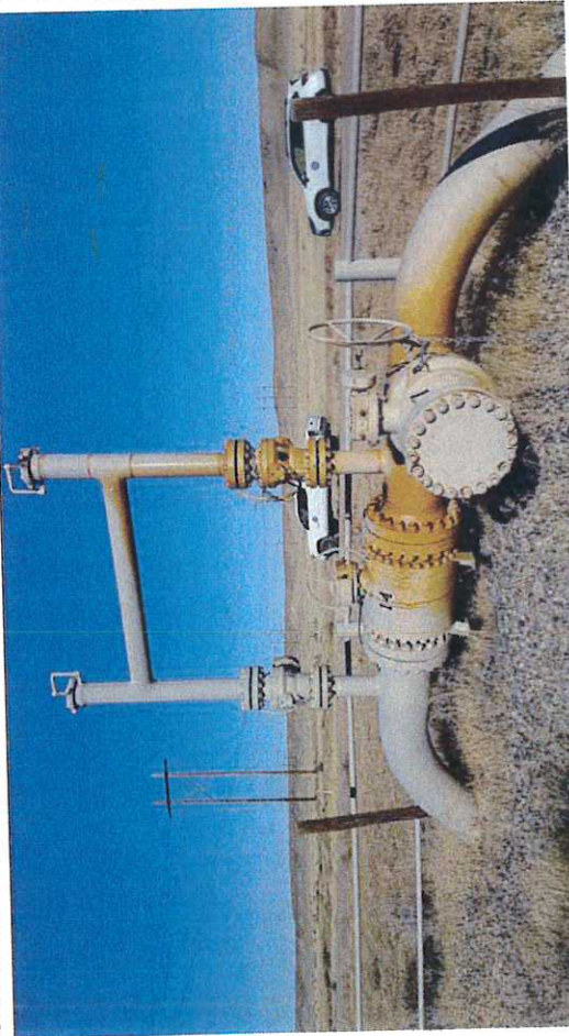
Picture #9: Block Valve assembly BV-14, BV-15, BV-16, and BV-17.
