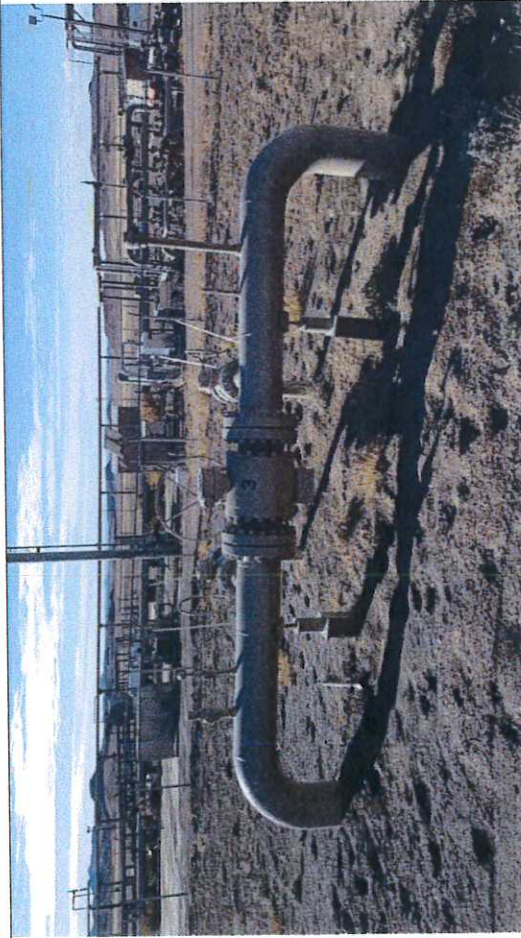
Picture #34: Observed valve assembly east of PEMC compressor station.
