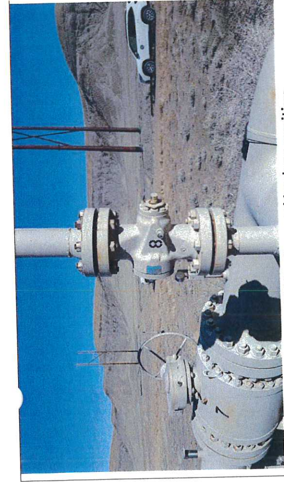
Picture #32: Block Valve BV-8, observed in close position.
