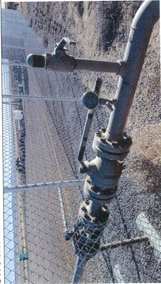
Picture #24: Observe Wesco Compressor Station at Blue Hills, PEMC Valve open position.
