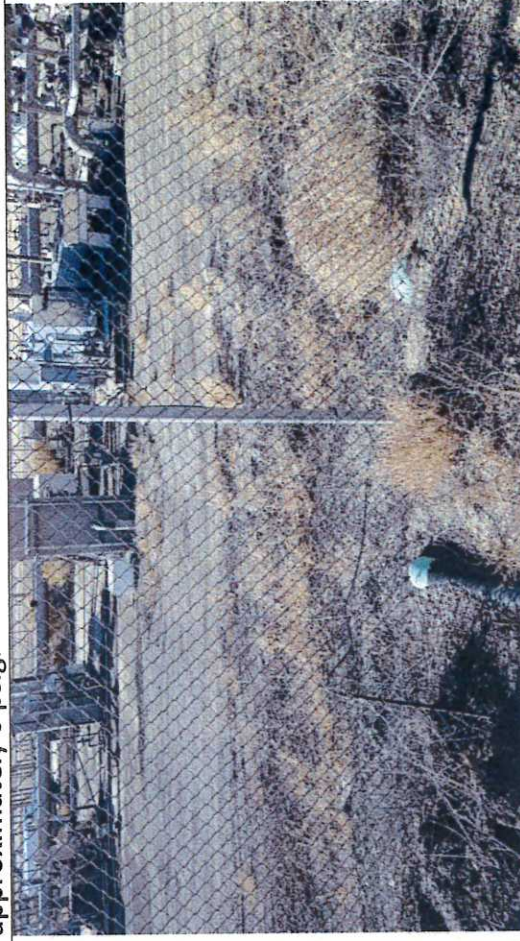
Picture #37: Observed PEMC compressor station exposed piping near the east fence.
