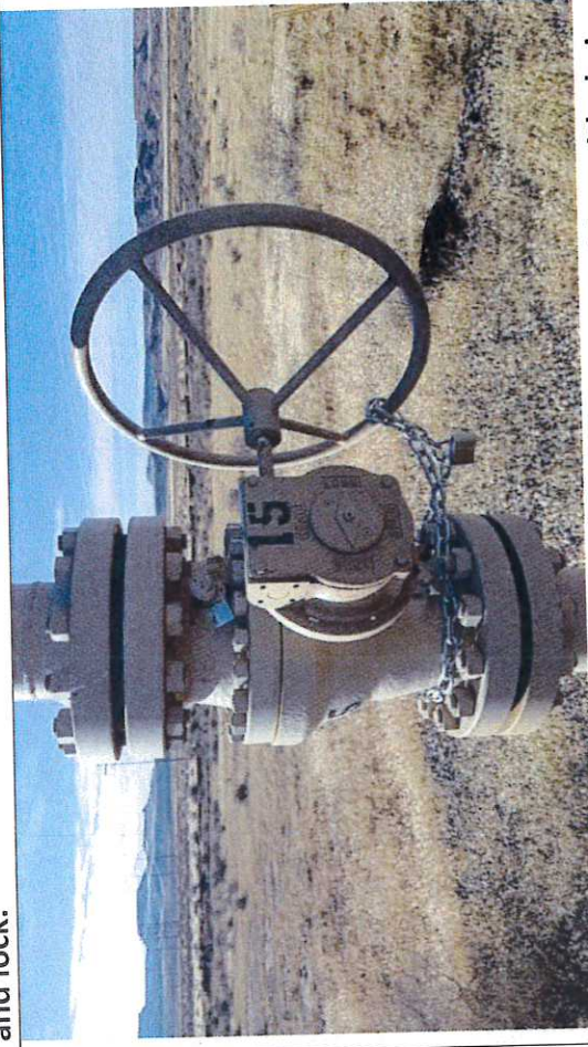
Picture #12: Block Valve BV-15, observed in close position with chain and lock.
