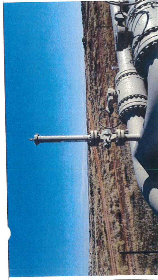
Picture #5: Block Valve BV-19 (Blowdown Vent), observed in close position.
