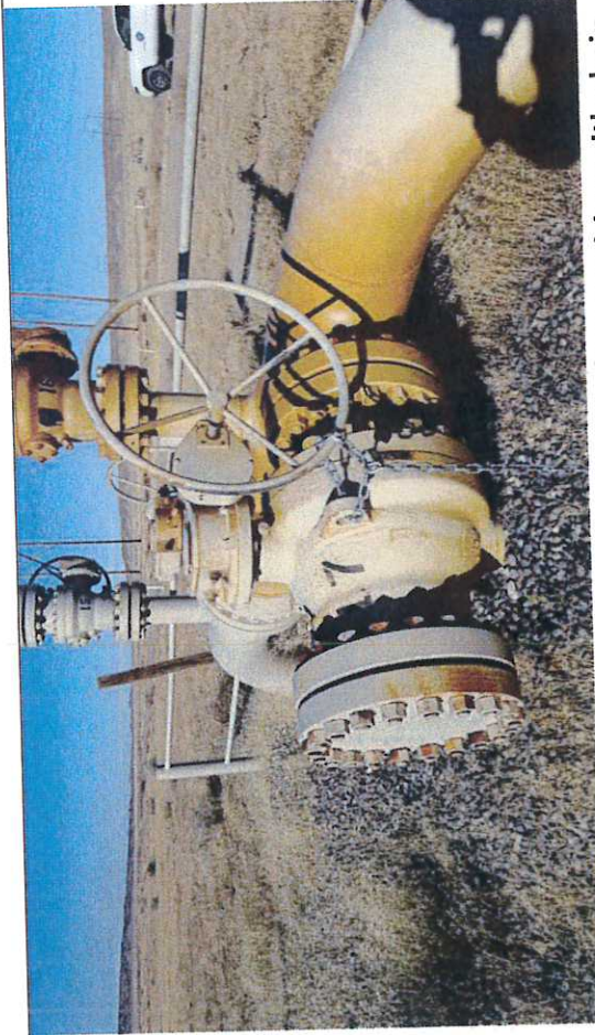
Picture #11: Block Valve BV-17, observed in close position with chain and lock.
