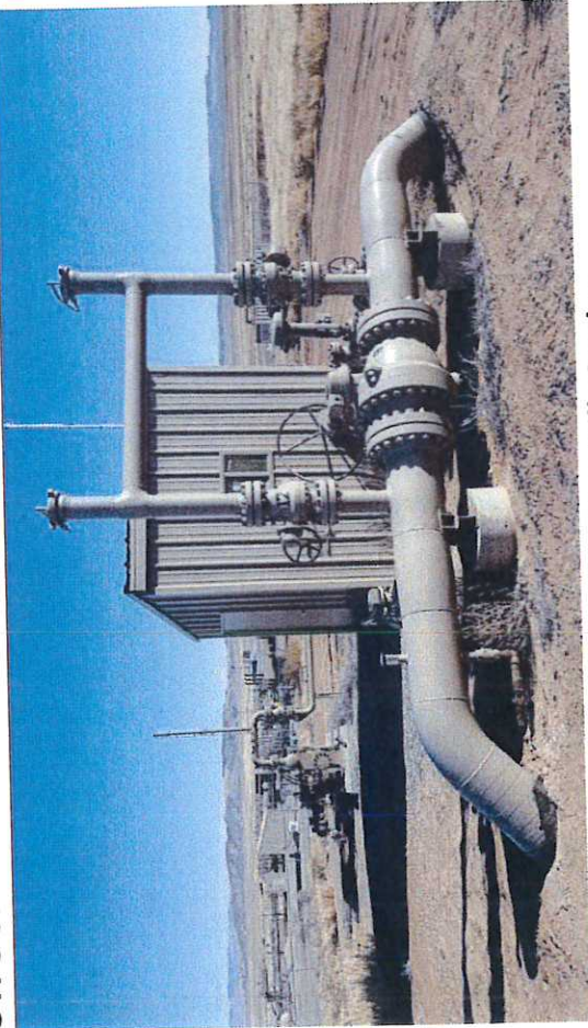
Picture #14: Wesco Tie-In Point at Blue Hills Station.
