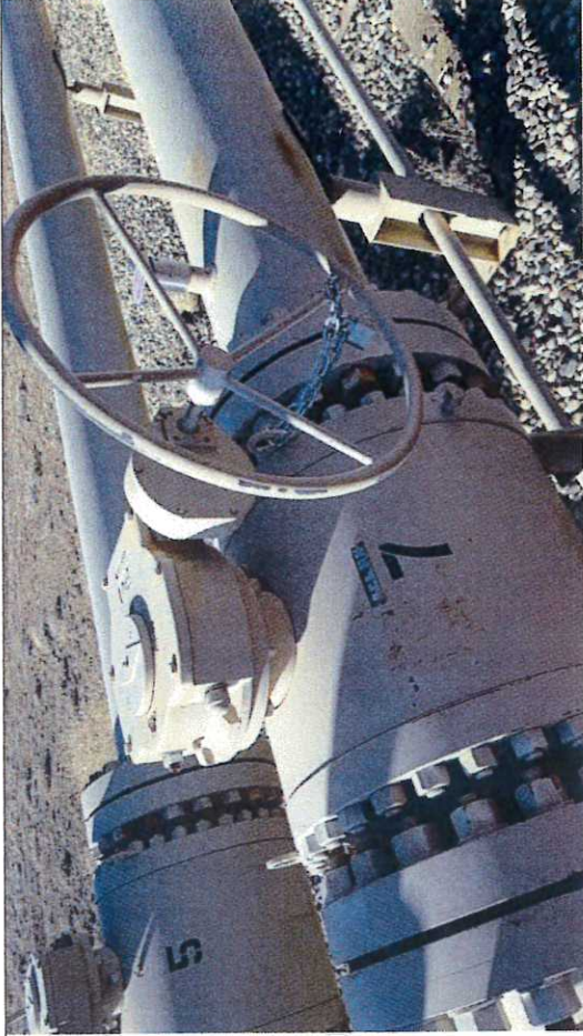
Picture #29: Block Valve BV-7, observed in close position with chain and lock.
