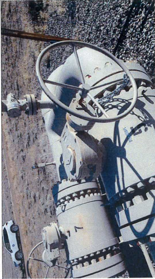
Picture #31: Block Valve BV-5, observed in close position with chain and lock.
