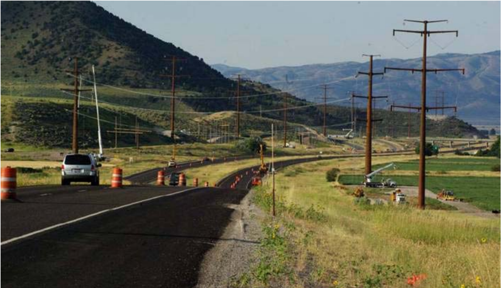
Populus to Ben Lomond – I-15 crossing south of Populus substation
