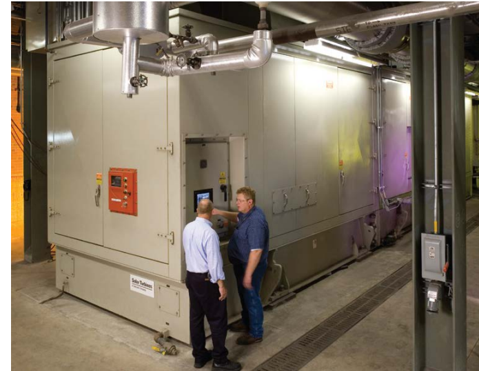
15 MW gas turbine generator set at Michigan State Univ., Solar Turbines Inc.
