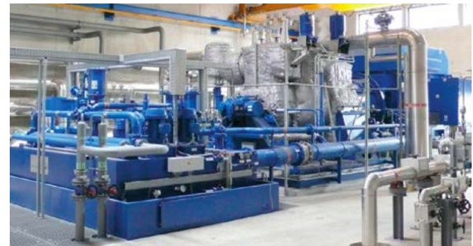
14 MW biomass system, courtesy of MAN Diesel & Turbo North America, Inc.
