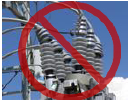
Figure 7—Incorrect Installation of Bushing Covers
