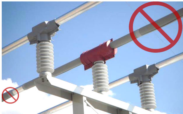
Figure 3—Incorrect Installation of Hose on the Entire Length of the Center Bus
