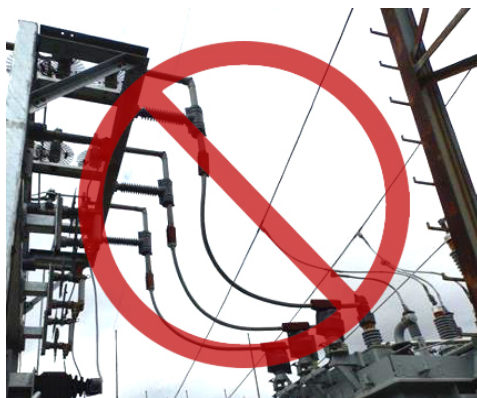
Figure 2—Incorrect Installation of Hose on the Entire Length of Conductor
