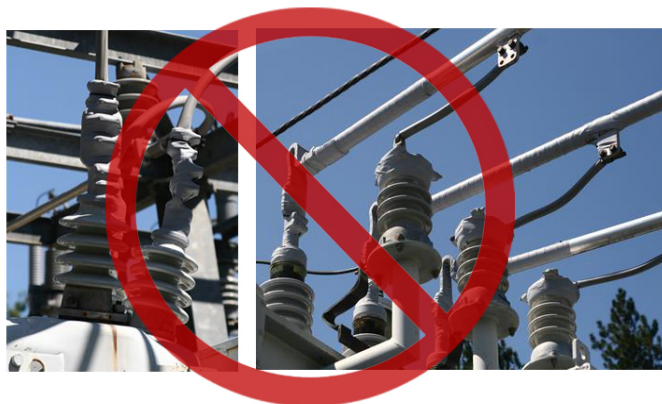
Figure 15—Inappropriate Use of Self-Adhesive Tape
