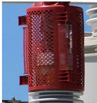
Figure 25—“Inspection” Bushing Cover to View Oil Indicator Window
