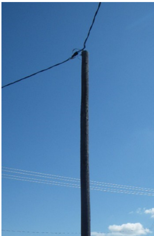
Figure 1—Secondary/Service Pole, Example
