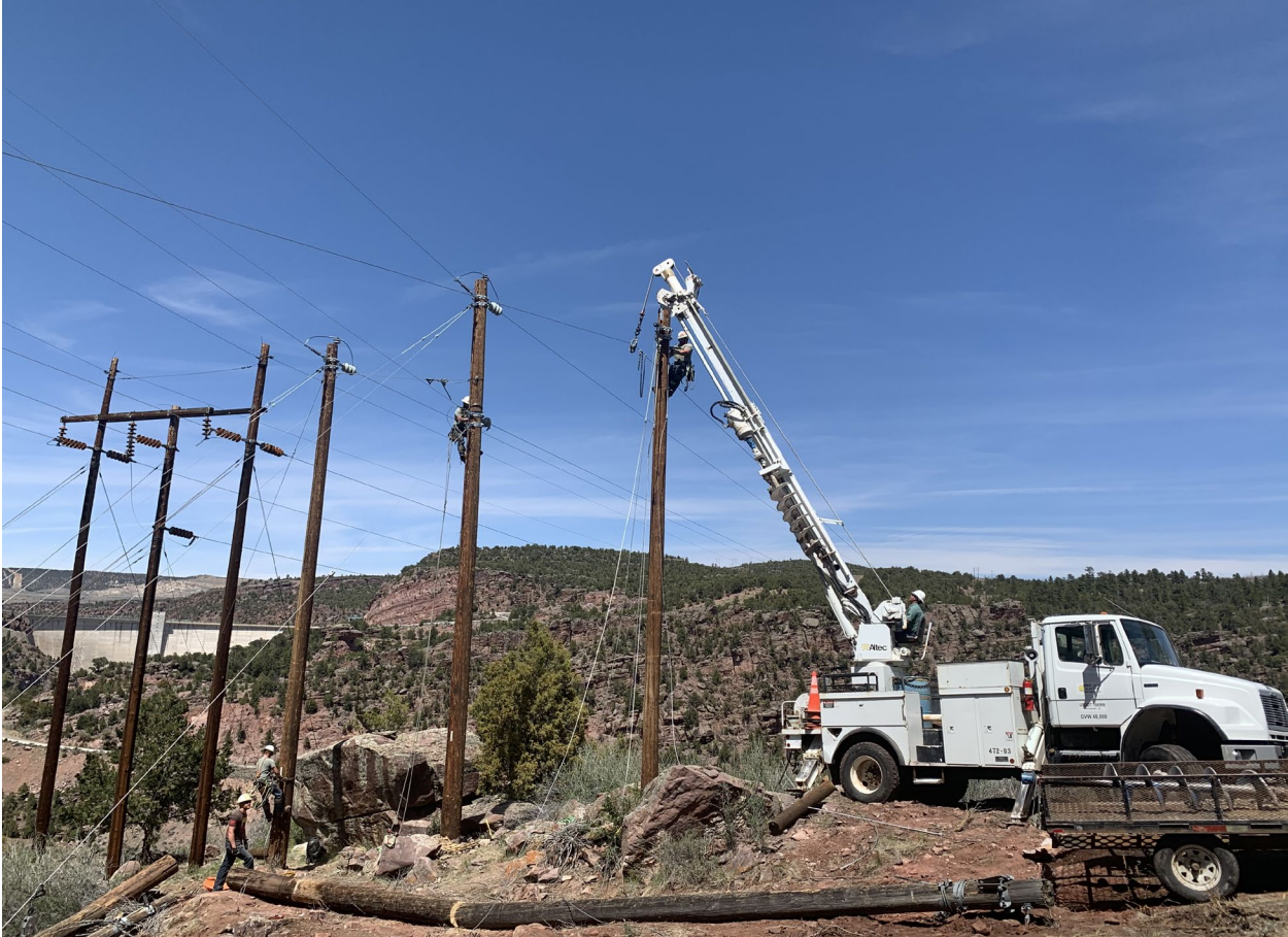
Figure 13. Changing poles to harden MLEA system 2020.
