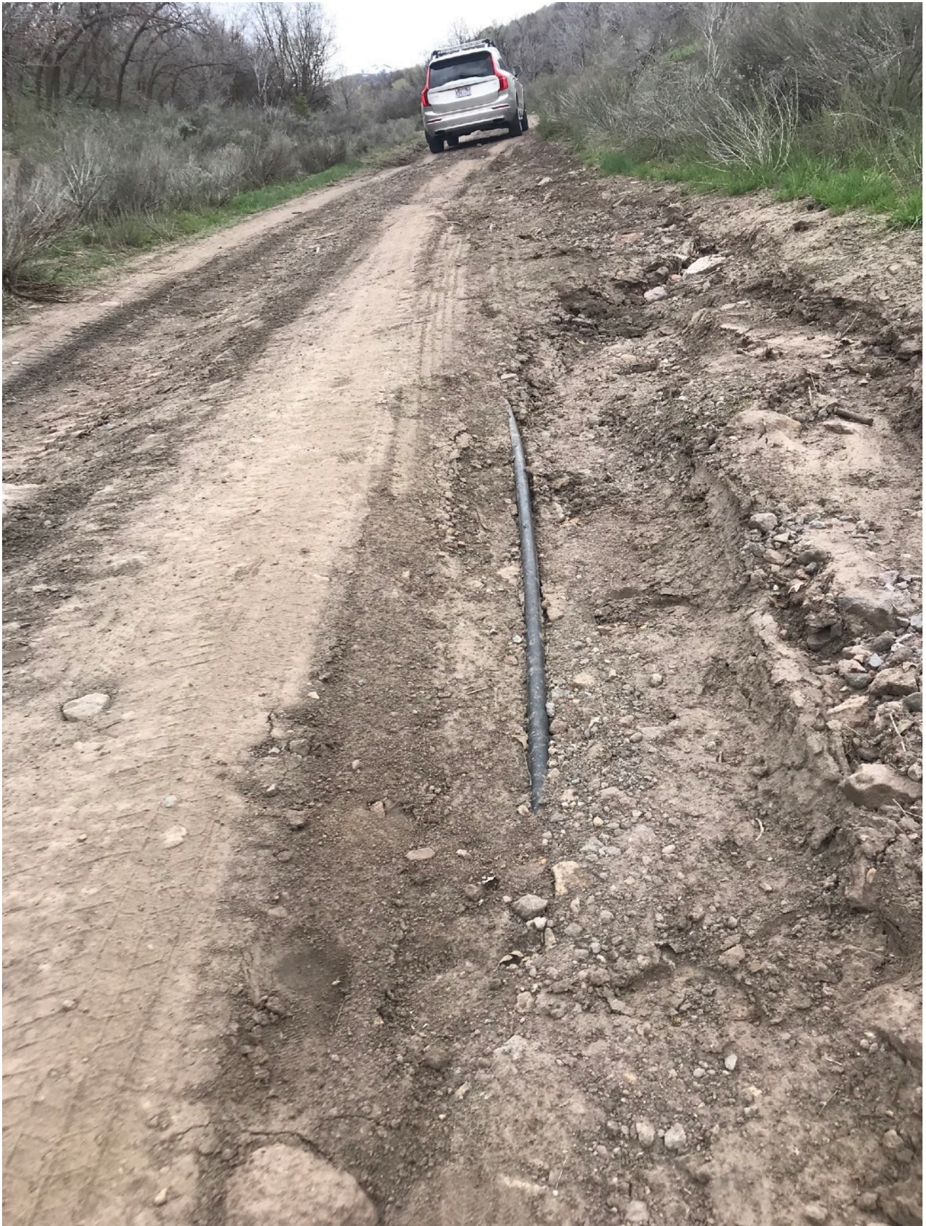
Photograph of the exposed 7200 volt power line approximately 194 feet above the first gate just above the parking area adjacent to the Yellow Fork Trailhead. Lat: 40°27'51.70"N, Long: 112° 5'7.40"W
