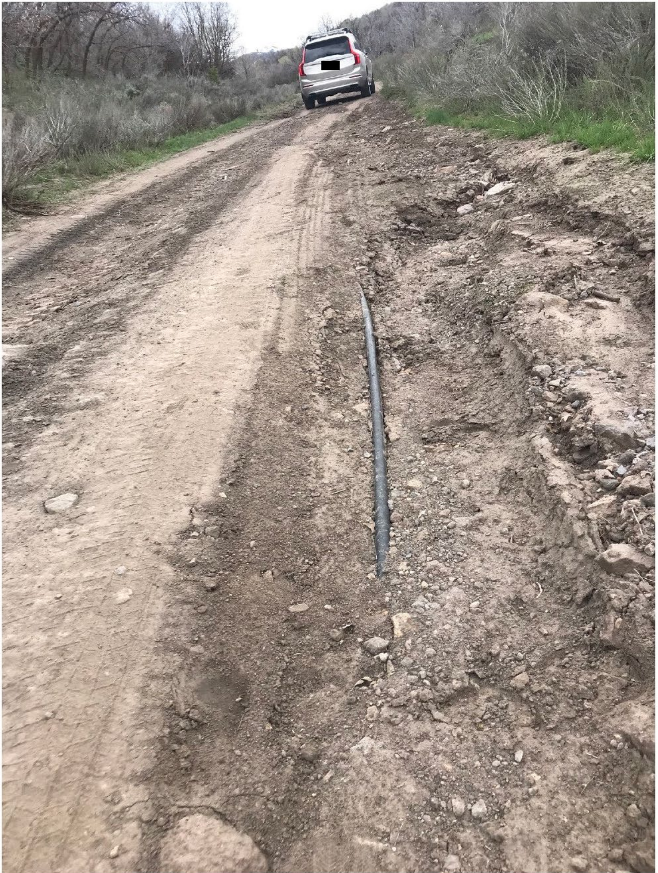
Photograph of the exposed 7200 volt power line approximately 194 feet above the first gate just above the parking area adjacent to the Yellow Fork Trailhead. Lat: 40°27'51.70"N, Long: 112° 5'7.40"W
