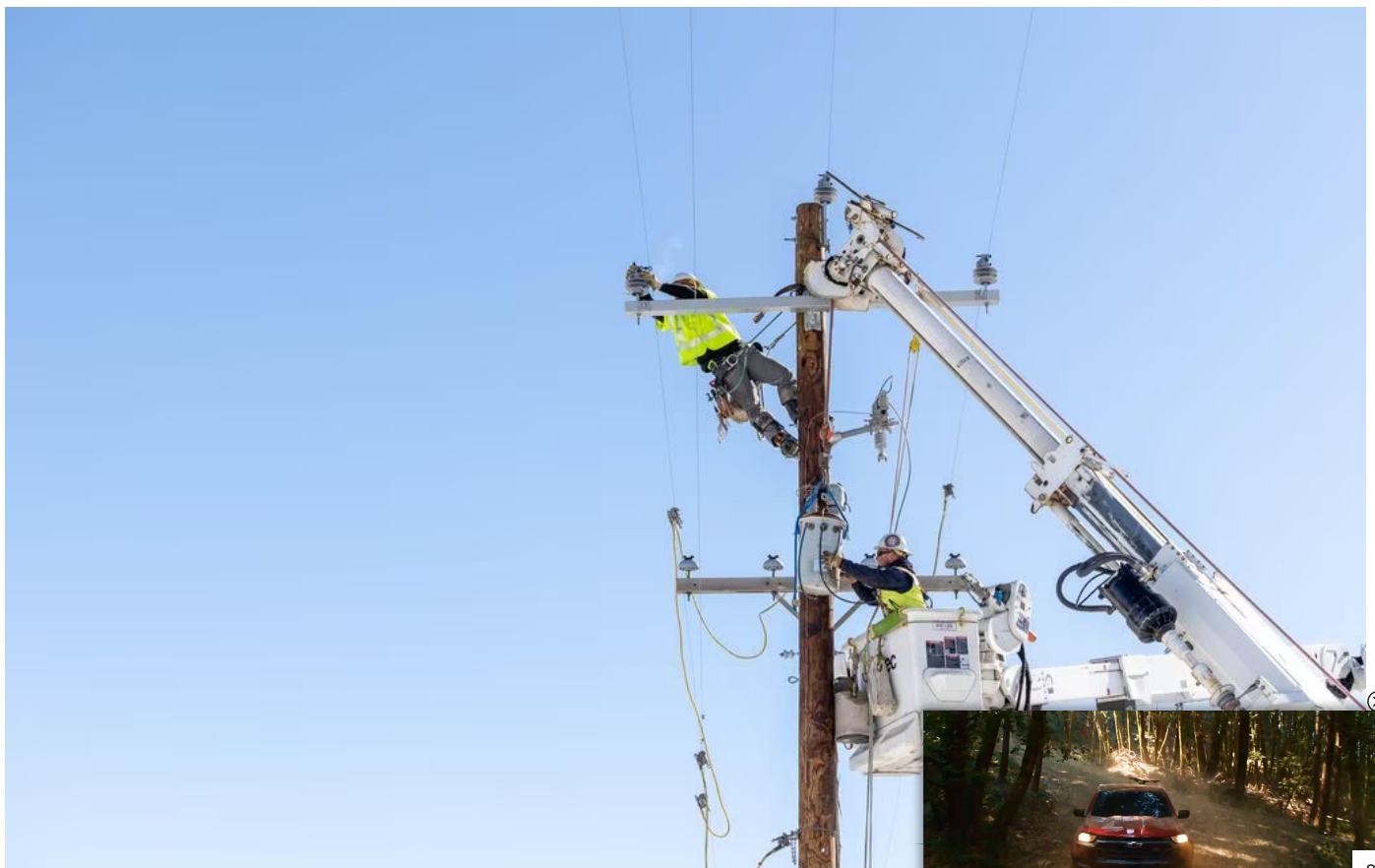
(Rocky Mountain Power) Crew near Mantua in Box Elder County updates a power line with "non-expulsion" fuses to lower
