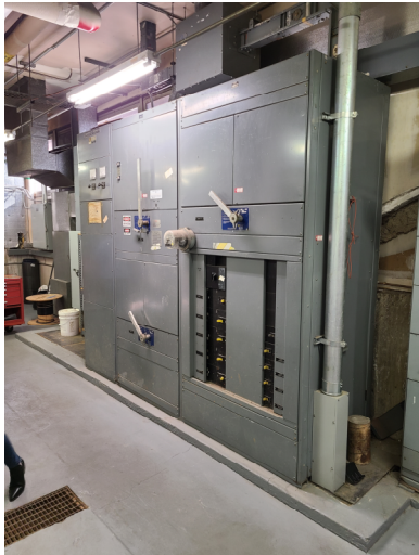
Existing Main 480/277V 3,000 A Switchboard
