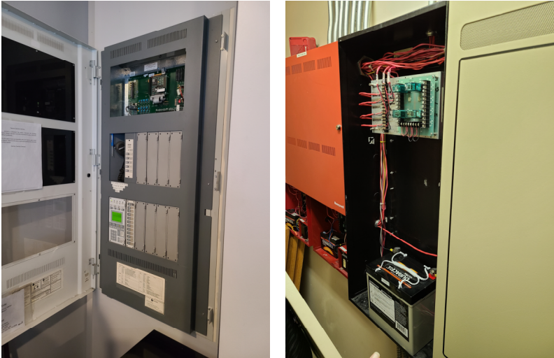
Existing Fire Alarm Control Panels and Battery Panels
