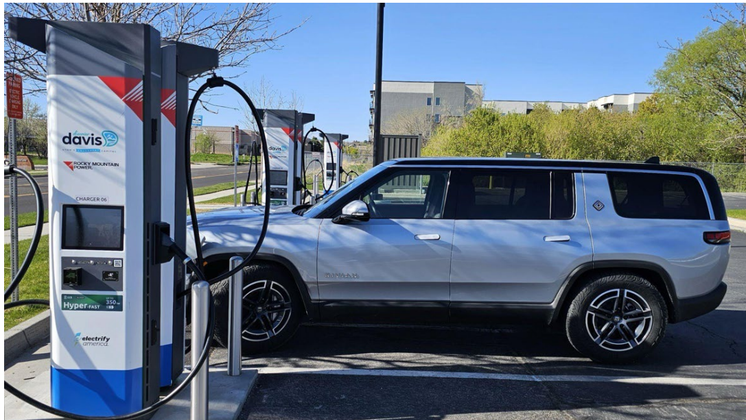
Figure 1. Newly installed Layton Chargers at the Davis County Conference Center
