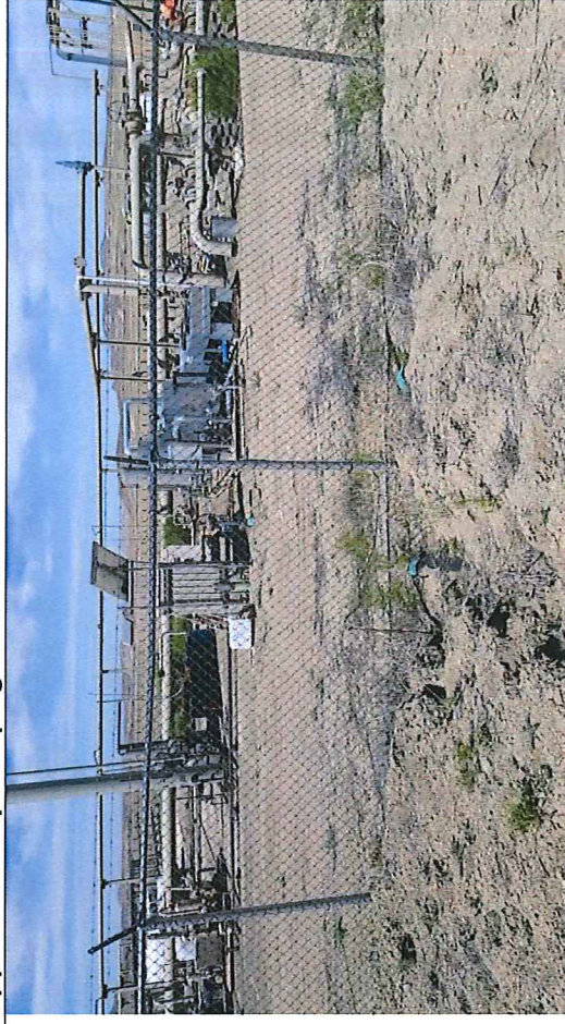
Picture #30: Observed PEMC compressor station exposed piping near the east fence.
