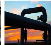
Interconnects with five interstate pipes and access to REX
